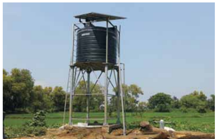
House Hold & Drinking Application at Sonapur, Odisha
