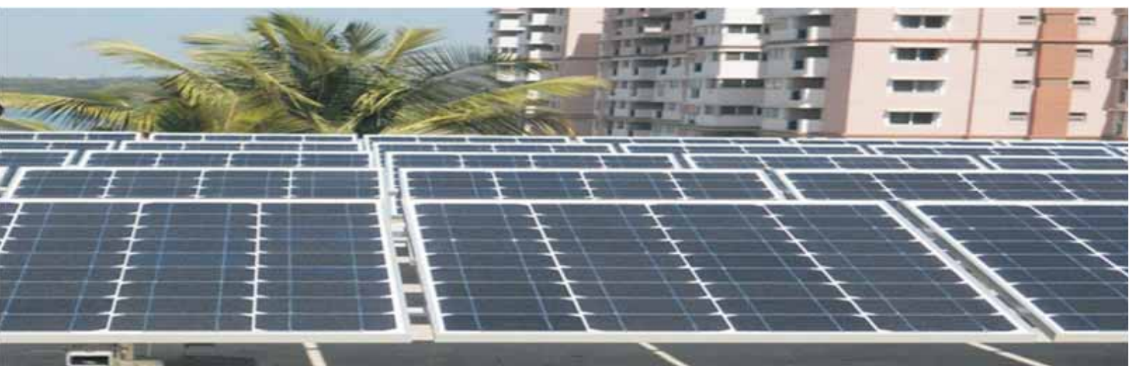
3.4 kW Setup of standalone Solar PV System with seasonal tilting of structure at Bangalore
